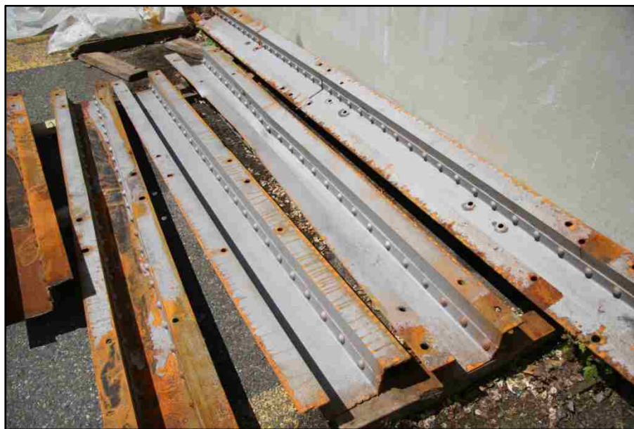
Figure 3.8 Guardrail Specimens after Sandblasting
